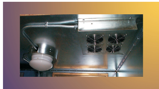
Light Fixtures and Exhaust Fans
